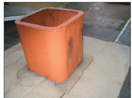
Damaged crown and eroded mortar joints should be repaired before relining.
