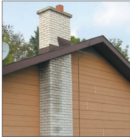
Stains like these are caused by condensation of moisture and creosote from cool flue gases.
